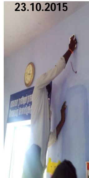
Electric Bell fixed at the Primary School, Thiruvadisulam- 23.10.2015
