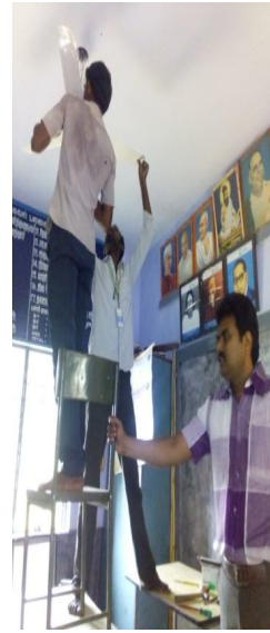
Fans fixed at Primary School, Thiruvadisulam- 23.10.2015
