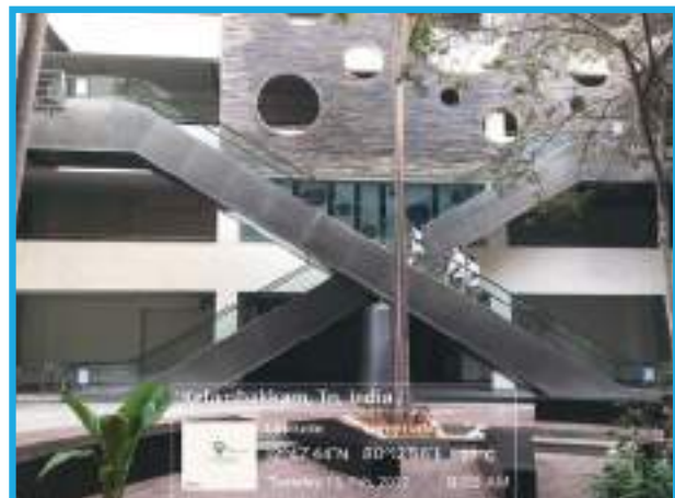
Escalator in College Block
