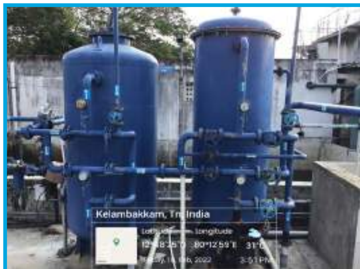
Water Softner Plant
