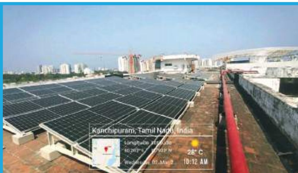
Roof Top Solar Power Plant
