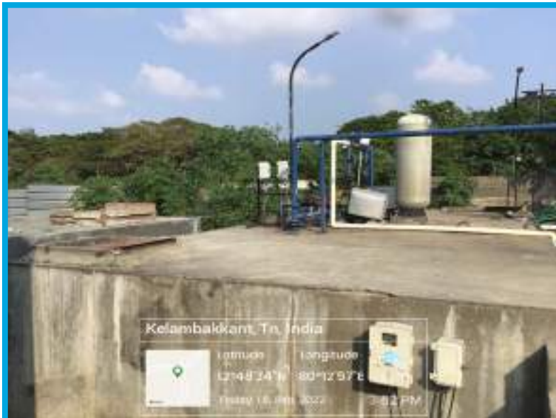
Soft Water Storage Tank
