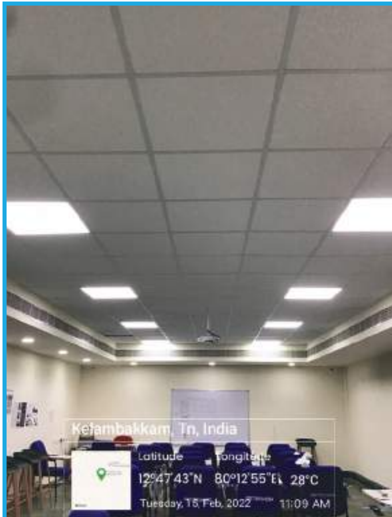
LED Lights in Classroom
