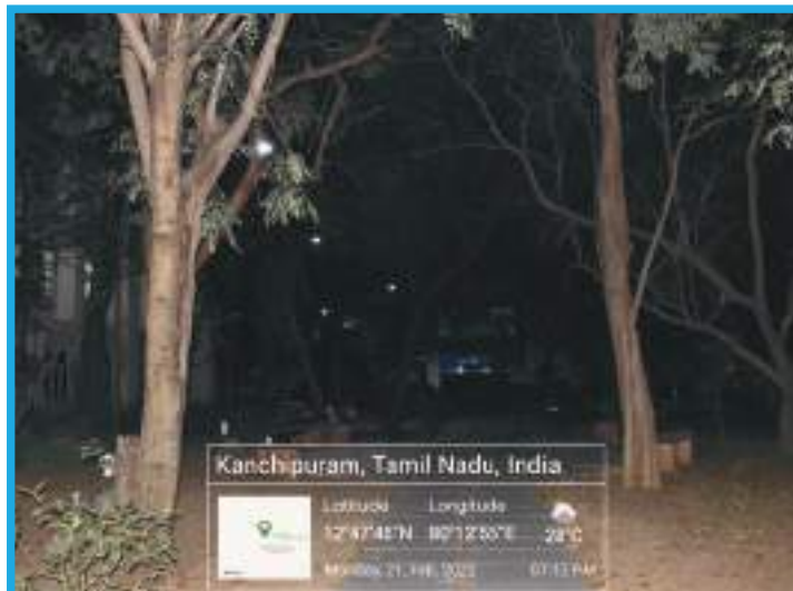
LED Street Lights at Night
