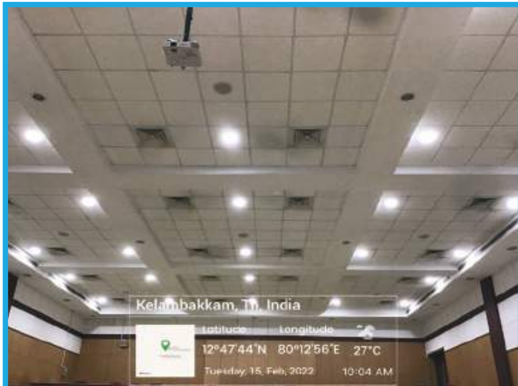
LED Lights in Lecture Hall
