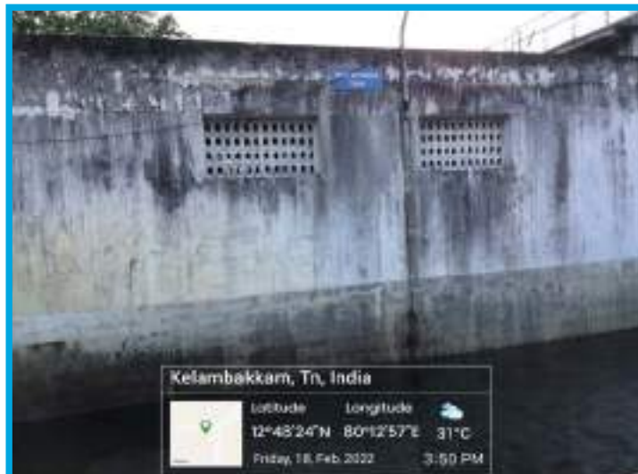
Treated Water Storage Tank
