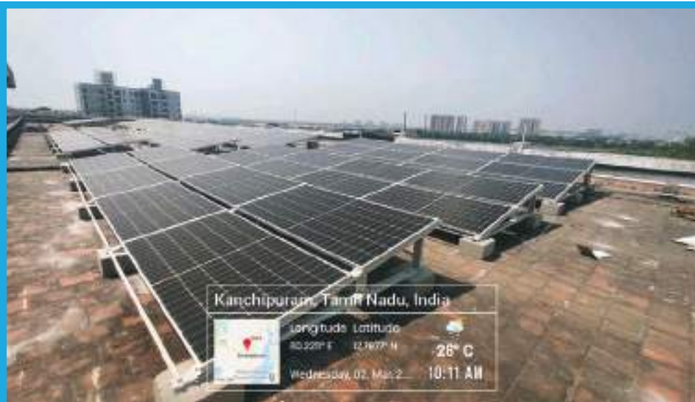
Roof Top Solar Power Plant
